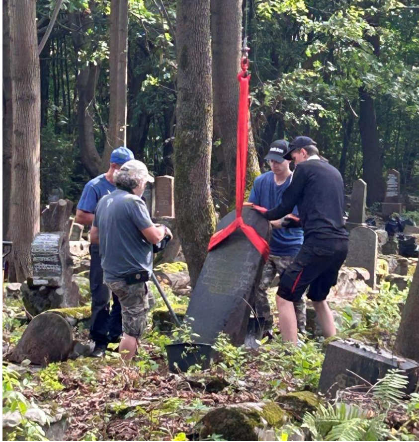
Josh Degen and local crane crew work in the newly cleared sections.
